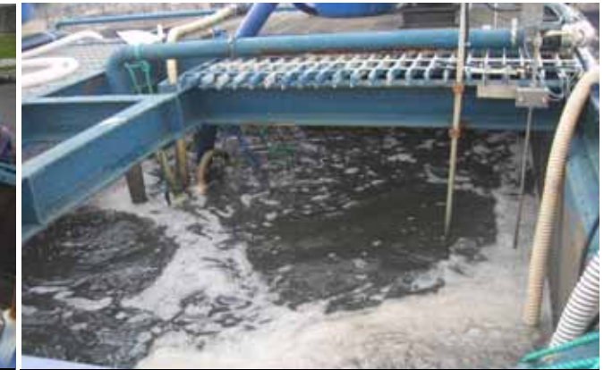
Stage 3 Anoxic Tank
