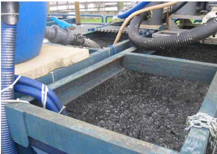
Stage 4 Anaerobic Tank
