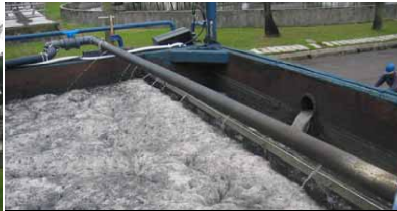
Stage 2 Influent entering into aerobic tank
